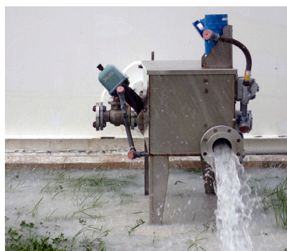
Continuous monitoring & control for floating roof tank drains
