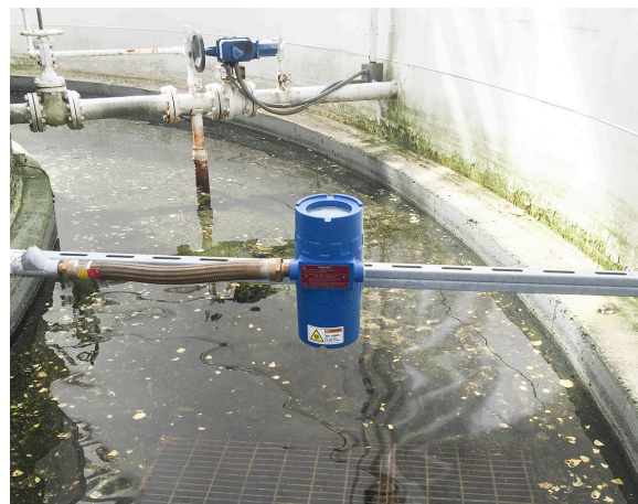
24/7 tank dike monitor with automated valve closure
